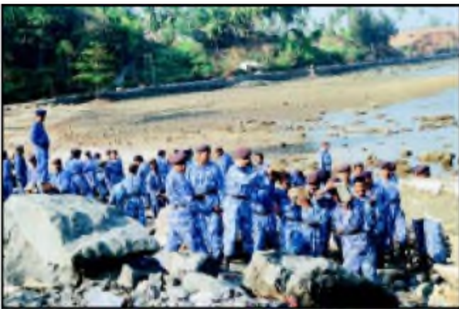
99 FAF personnel repairing Culvert Road near sea, South Poir, Port Blair (A & N), India
