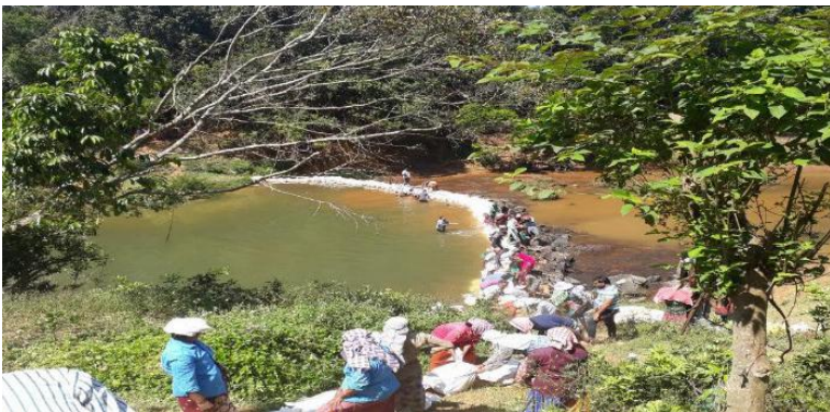
Construction of a check dam following a flood in Wayanad district in Kerala in 2019
