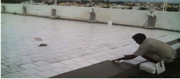
Installing white cooling tiles on a roof of a building in Tamil Nadu
