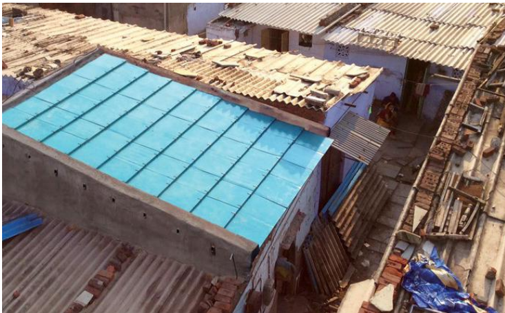
Modular panel roofs are replacing metal sheeting and poor quality cement in a slum in Ahmedabad, Gujarat
