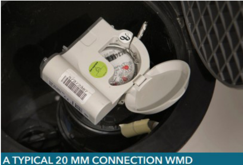
Fig. 10 shows two images of the Water Management Devices. 61
